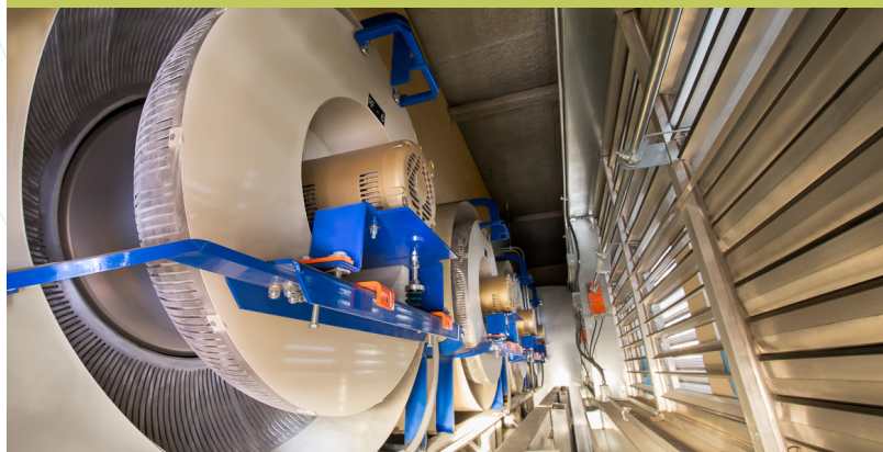
▲ AcoustiFLO penthouse site erected exhaust array
